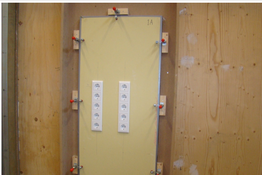
Picture B.1 General overview electrical outlets
